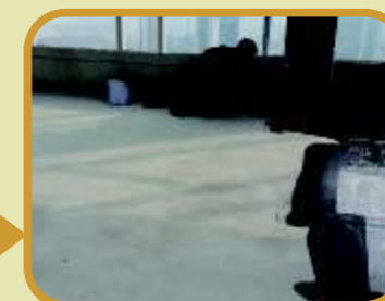
Joint strength treatment: Joint parts(Such as Impinges mouth, Wear plate pipelines, internal and external corners, etc.) treatment by rubber bitumen waterproofing coatings
