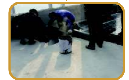
Paving the self adhesive membrane: Removing the isolation film of the membrane's lower surface before the coating cooled, then paving the membrane on the coating layer.
