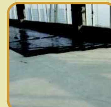
Test Paving the waterproofing membrane: Paving the waterproofing membrane on the substrate after the primers dried, and then rollback after confirmed the position.
