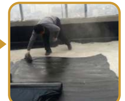
Applied the rubber bitumen waterproofing coating: Pouring the heated coating into the specialized scale bucket, and the coating weight is 11.5kgs of each bucket, then pouring 11.5kgs of coatings onto each grid separately, to ensure the coating dosage is 2.5kg/m 2 . Brushing the coatings on the substrate evenly according to the snapping line ranges.
